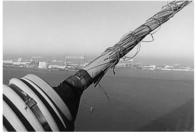
Figure 4. Broken stay cable (32 downstream) at the Saint-Nazaire Bridge.
