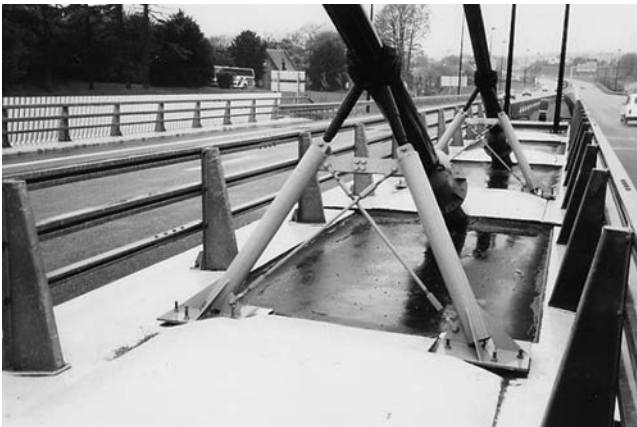
Figure 45. A damper at the Iroise Bridge over the River Elorn.
