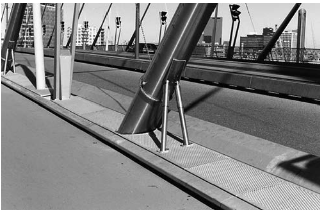
Figure 47. Example of dampers installed too close to the anchorage, which could not prevent cable vibrations.
