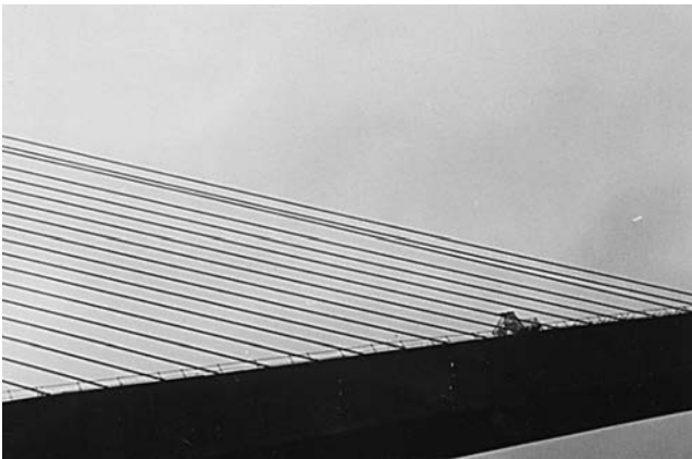
Figure 2. Stay cables of the Brotonne Bridge when vibrating during construction (photo courtesy of J. Combault).
