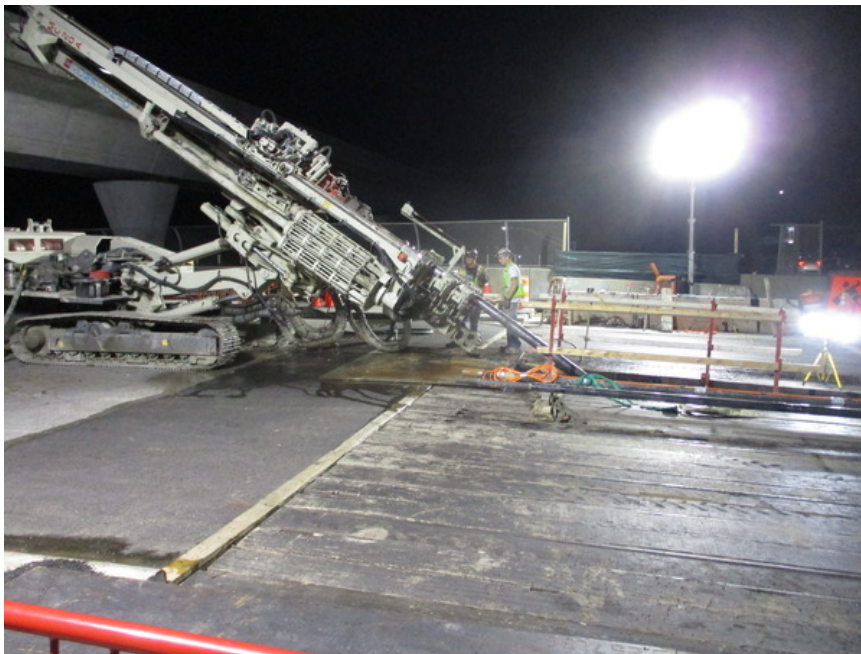
Figure 13. Photo of tiebacks being installed during overnight operations at the 109 th Avenue Bridge west abutment, looking south. Note the temporary deck panels which have been partially removed to allow for the work to take place during overnight closure windows.
