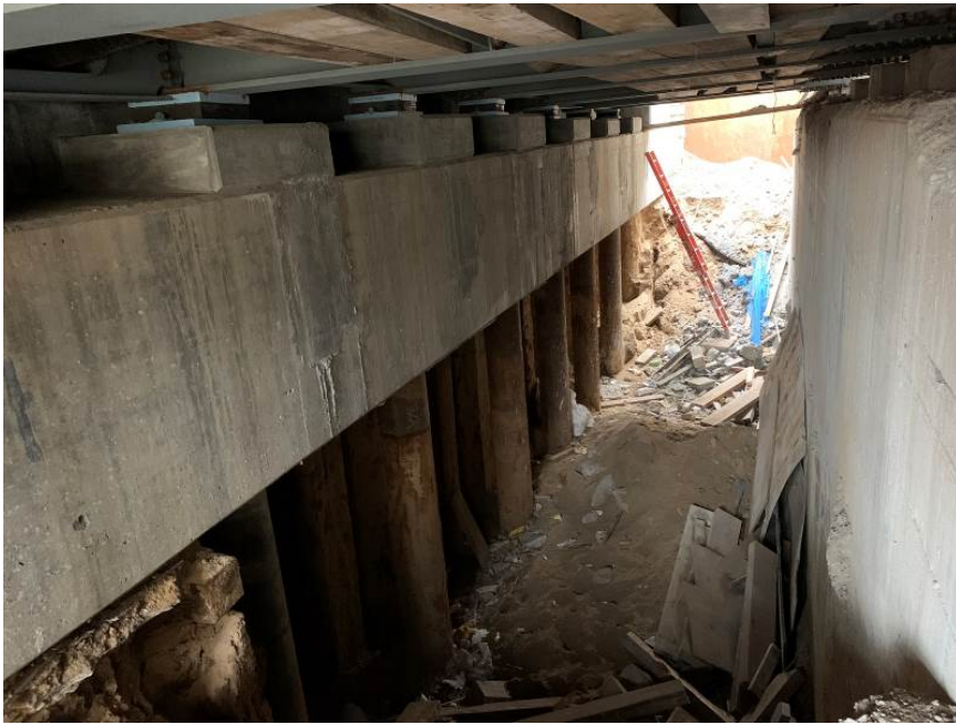
Figure 8. Excavation between the new abutment pile cap (left) and existing abutment (right). View of the 133 rd Avenue Bridge east abutment, looking south.
