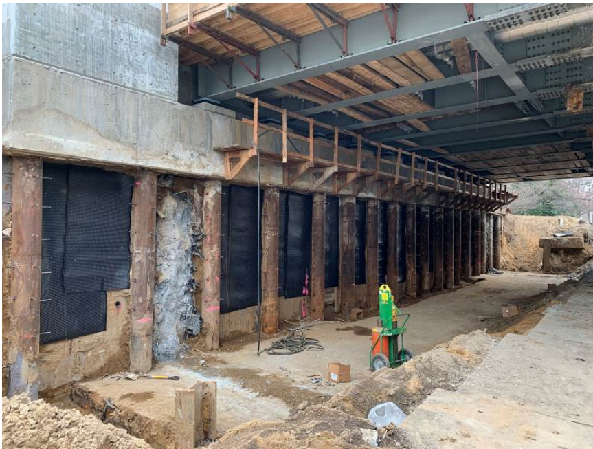
Figure 9. View of the new Foch Avenue Bridge east abutment, looking south, after the removal of the existing abutment.
