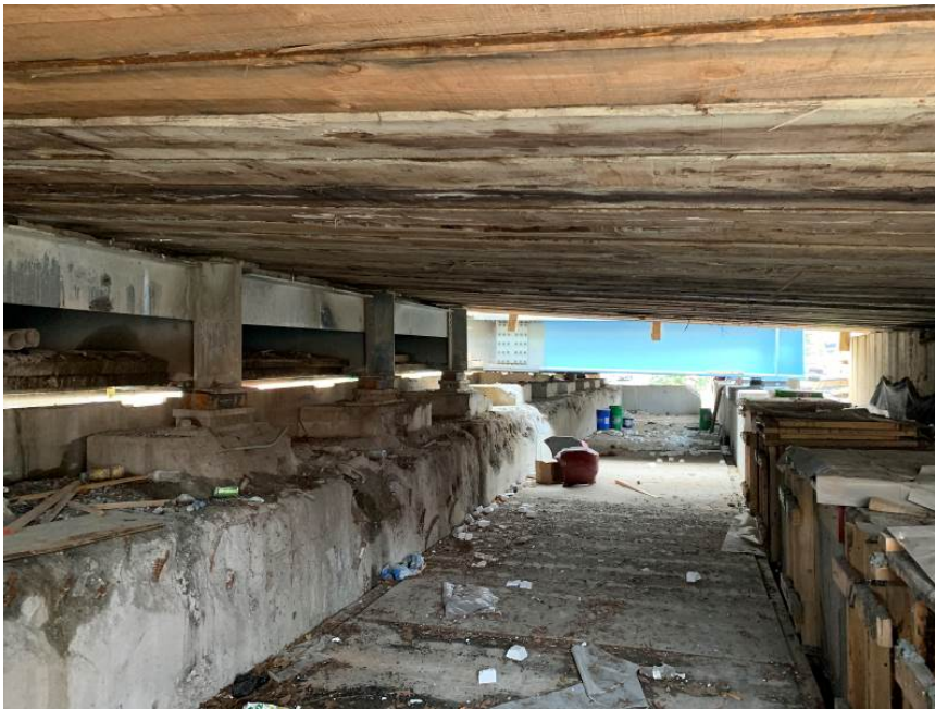
Figure 5. Temporary timber deck panels (above) spanning the gap between the existing abutment (left) and the new abutment pile cap (right). View below deck at the 109 th Avenue Bridge east abutment, looking north.
