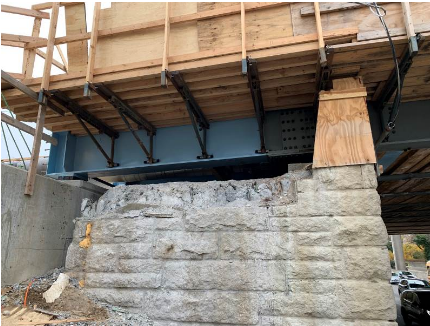
Figure 7. Stringer extensions installed between the existing abutment (right) and the new abutment pile cap (left). View of the 109 th Avenue Bridge east abutment, looking south.
