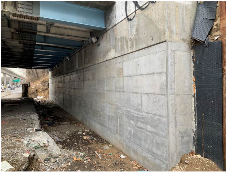
Figure 10. Completed new fixed frame abutment with wall facing. View of the 109 th Avenue Bridge west abutment, looking south.
