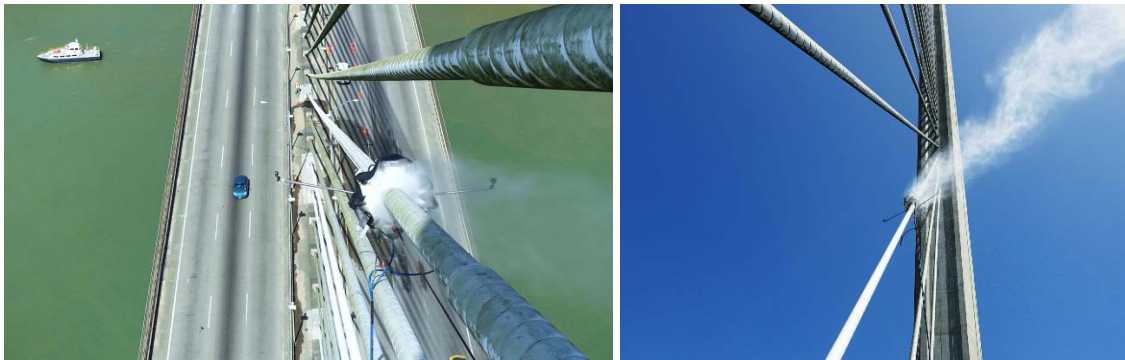
Figure 10. High-pressure cleaning device travelling along a stay cable of Puente Centenario, Panama, 2018. Left: View from pylon to bridge deck. Device being pulled upwards. Right: View from bridge deck to pylon. Clearly recognizable difference between cleaned white stay pipe and non-cleaned stay pipes.
