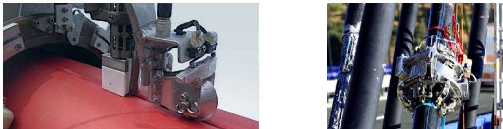
Figure 8. Semi-automated welding for PE repair works of stay pipes. Left: Detail of PE extruder in front of the device. Right: Device welding a longitudinal welding seam at Puente Ingeniero Carlos Fernández Casado, Spain, 2016.
